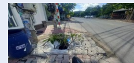
Figure 8: A drain cover has a crack in the middle of it in real life
