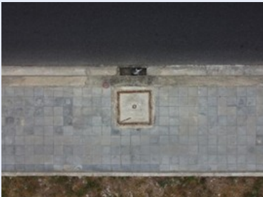
Figure 12: An example of hypothetical case of drain cover having a line crack
