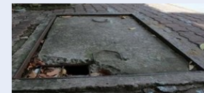
Figure 7: A drain cover is cracked at the corner in real life
