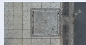
Figure 9: A drain cover has a line crack in our campus in Thu Duc city, Vietnam
