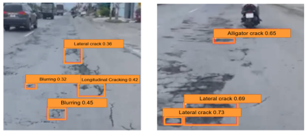
Figure 9: The results identifies several images of damages Pictures made by the RTI IMS model, "Source: The authors".
